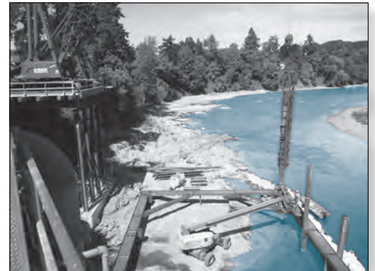
The framework for a temporary work enclosure, called a cofferdam, goes into place at the river intake pump station. Once constructed, water will be pumped from the enclosure to create a dry construction zone within the riverbed.
